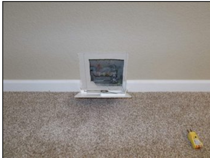
35. Main water shut off basement front
