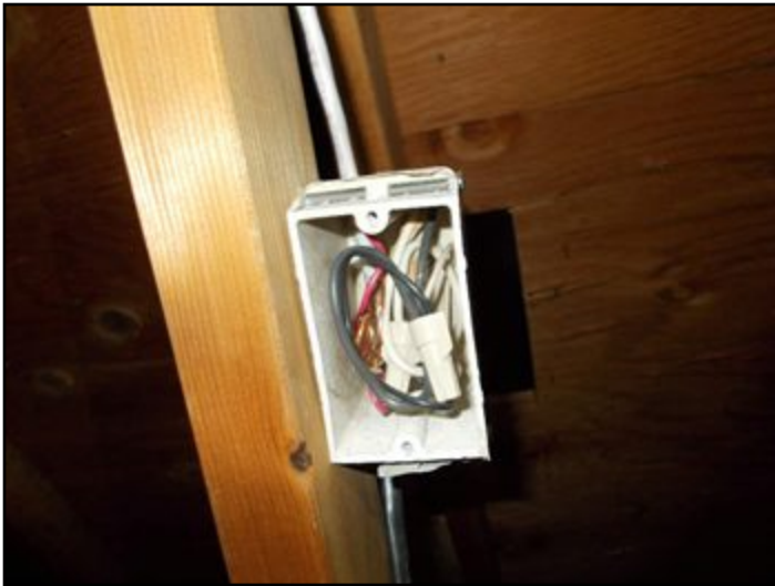
24. Cover loose or missing
