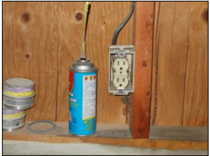
25. Cover loose or missing
