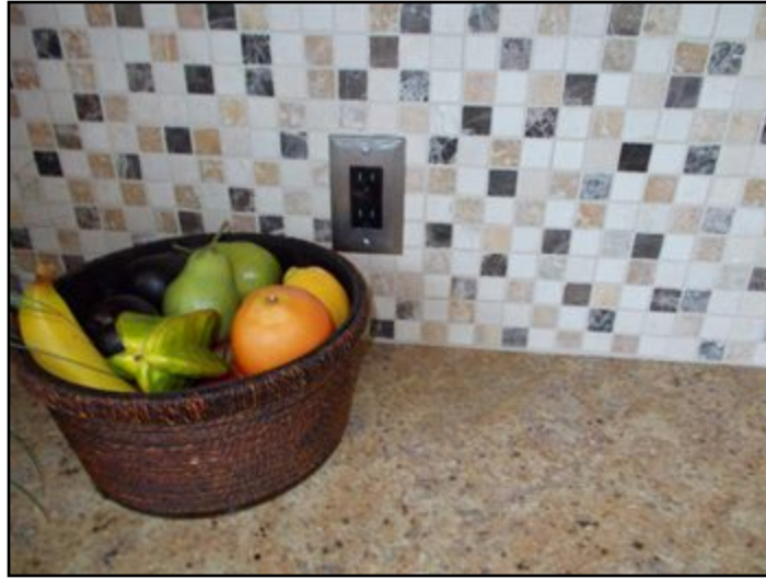
26. No GFCI (Ground Fault Interrupter)
